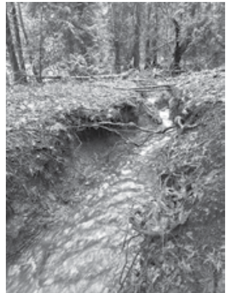
Stream bank erosion in Shingle Creek, adjacent to the Masthead Crescent/Shingle Bay trail on North Pender Island. Photo by Erin O’Brien
